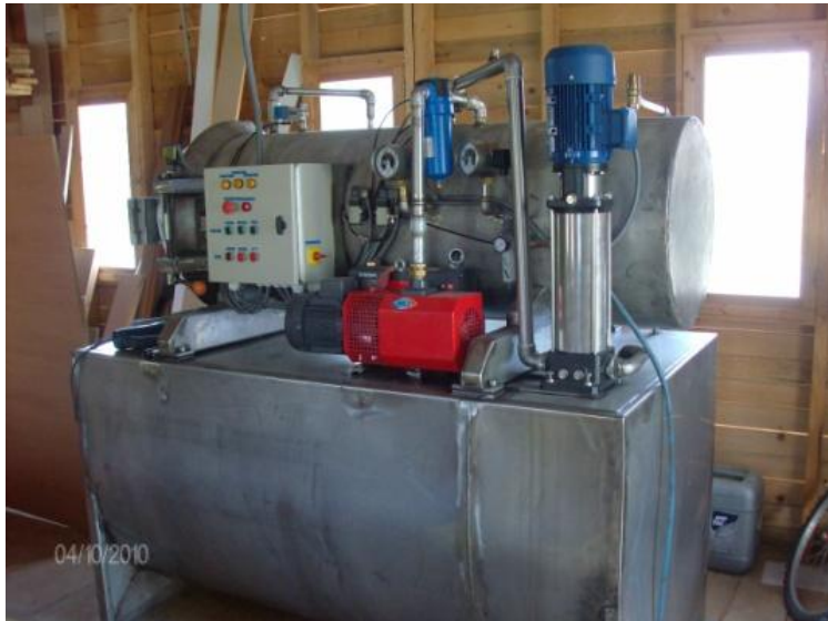
View of the wood-impregnation pilot plant (600 L) at WST
